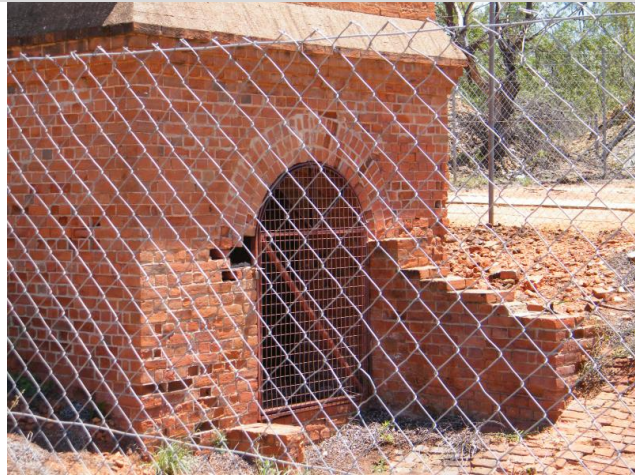
Base of the brick chimney stack showing safety mesh grill and current condition.
