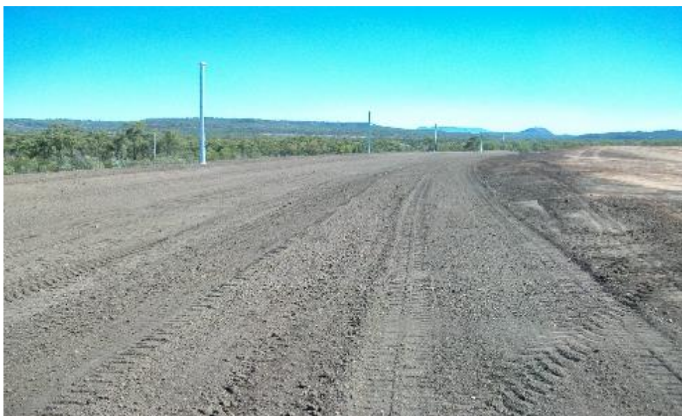
Figure 4-1: Rehabilitation Works at Dysart Landfill. Note landfill gas passive vents
