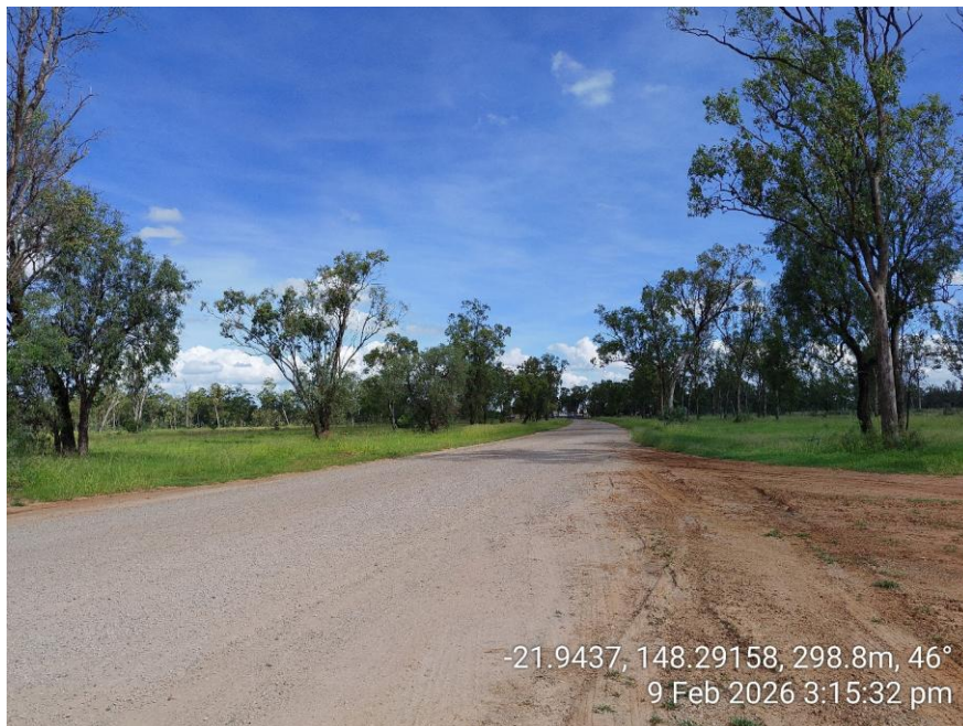
Figure 2: Condition of Poitrel Road (Chainage 70m)
