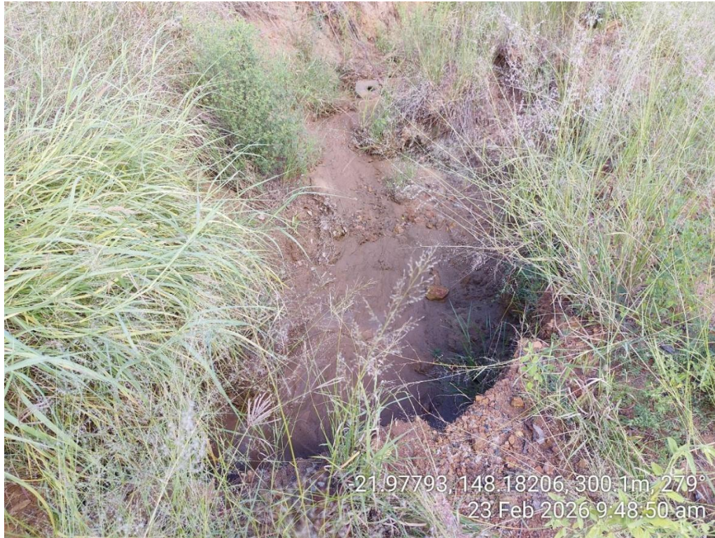
Figure 5: Chainage 1.52 (Current Safety Hazard)
