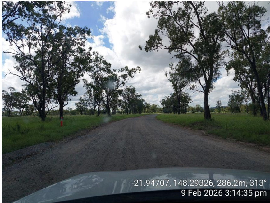
Figure 3: Condition of Poitrel Road (Chainage 480m)
