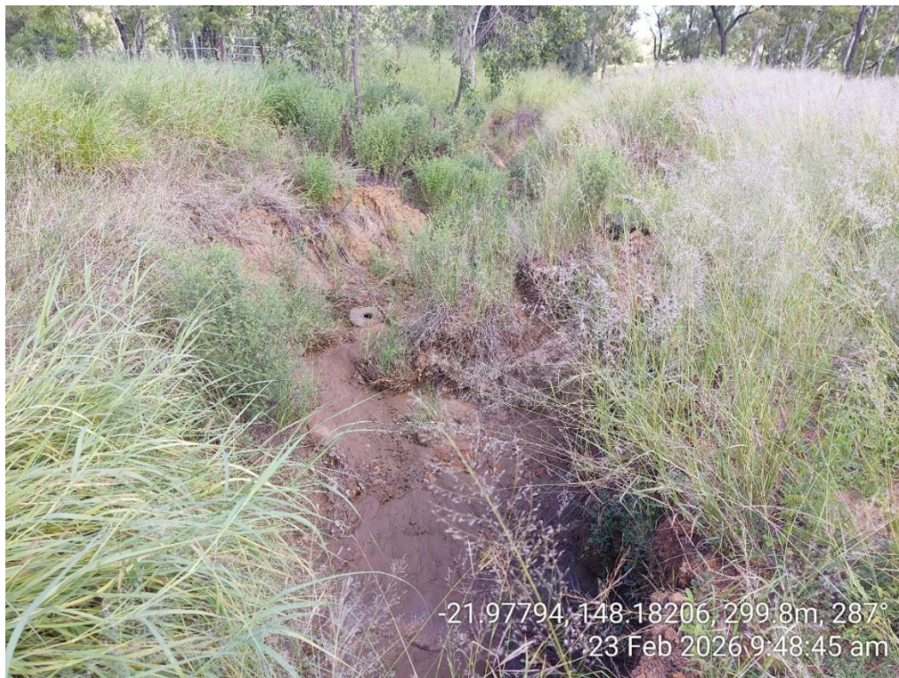
Figure 6: Chainage 1.52 (Current Safety Hazard)
