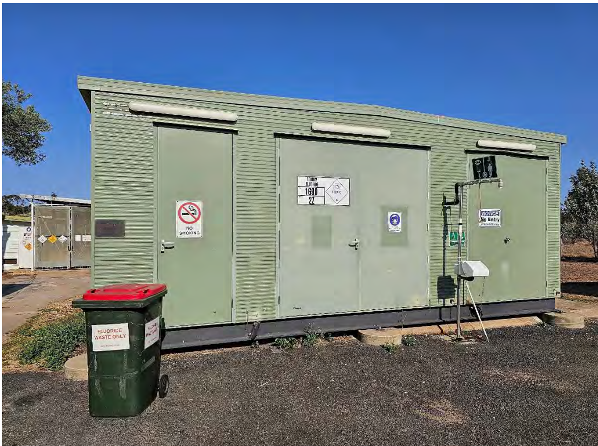
Photo 36: Tieri WTP Fluoride Building
