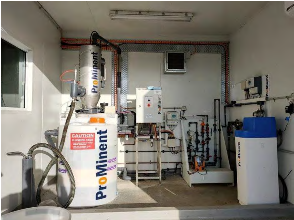
Photo 37: Tieri WTP Fluoride Dosing System
