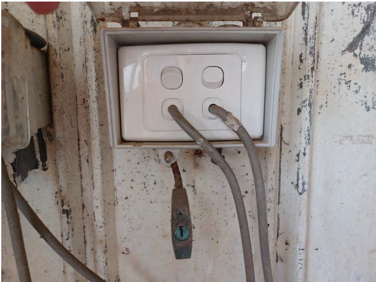
Photo 30: Moranbah WTP Dosing Pumps Hardwired – Compliant with Code of Practice Item 3.8.3
