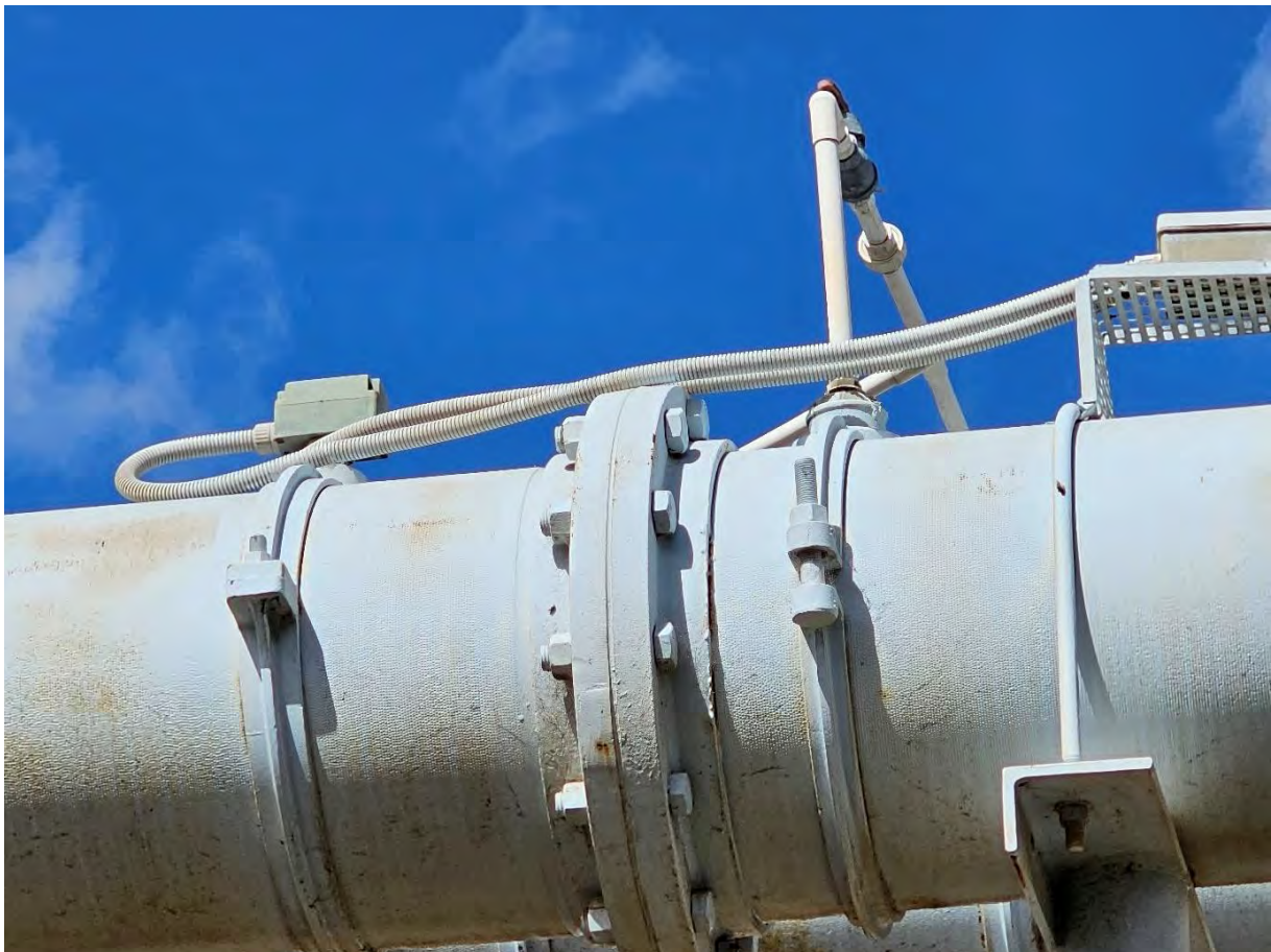
Photo 27: Moranbah WTP Filtered Water Pipeline Flow Switch – Compliant with Code of Practice Item 3.4.7
