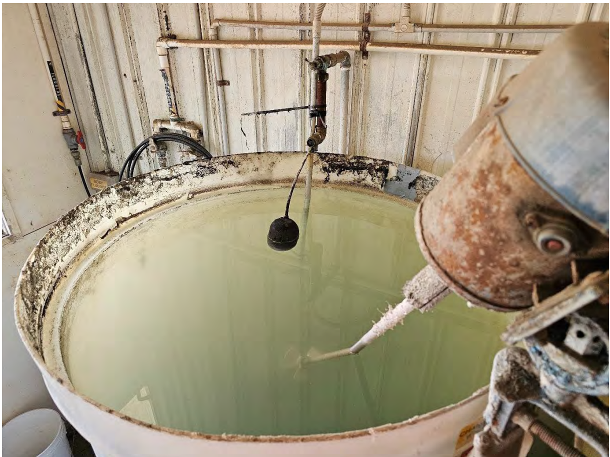
Photo 15: Fluoride Batching Tank Mixer
