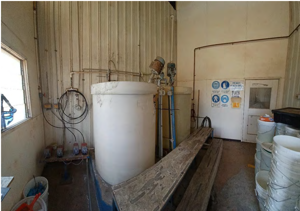
Photo 24: Moranbah WTP Fluoride Batching Room – Compliant with Code of Practice Item 3.2.7
