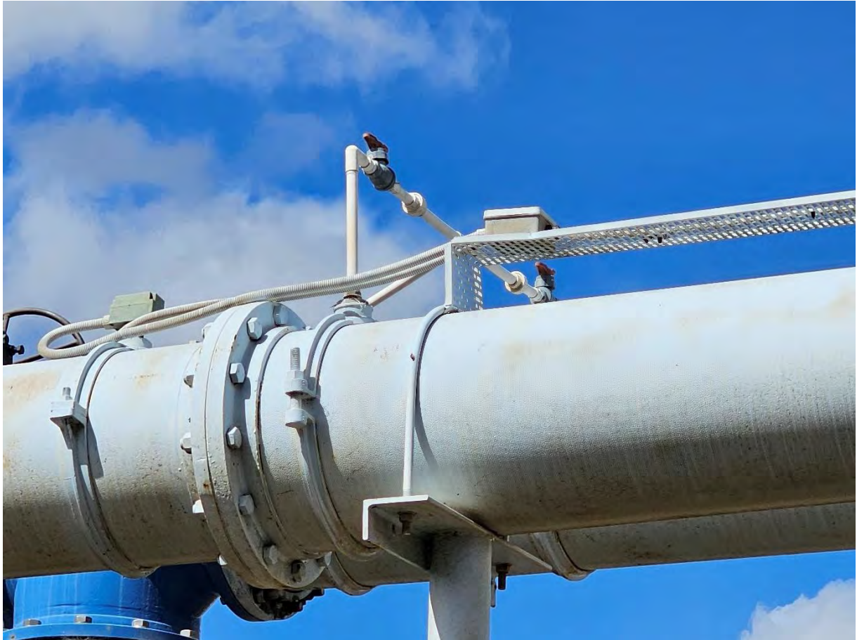
Photo 3: Moranbah WTP – Main Plant Flow switch and Fluoride Dosing location
