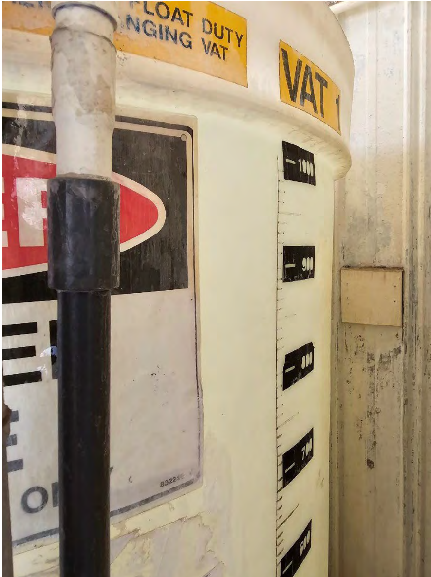
Photo 32: Moranbah WTP Fluoride Dosing System Graduated Lines – Compliant with intent of Code of Practice Item 4.6.12
