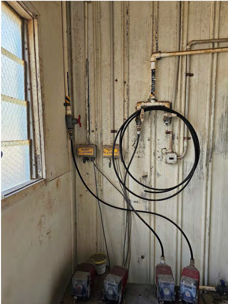
Photo 25: Moranbah WTP Conduit Labelling – Compliant with Code of Practice Item 3.2.11
