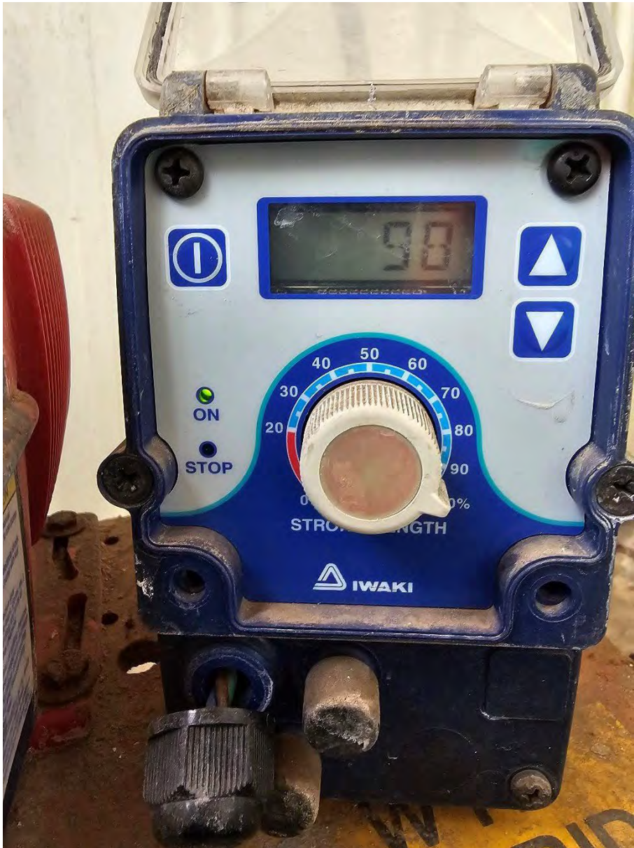
Photo 28: Moranbah WTP Fluoride Dosing Pumps – Compliant with Code of Practice Item 3.5.3
