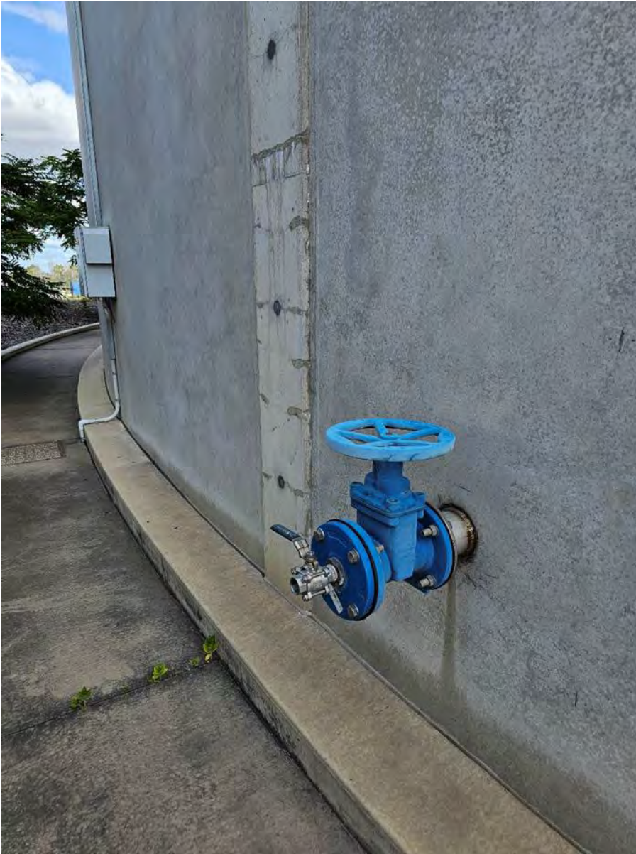
Photo 4: Moranbah WTP Reservoir No. 2 – Fluoride Sampling Location
