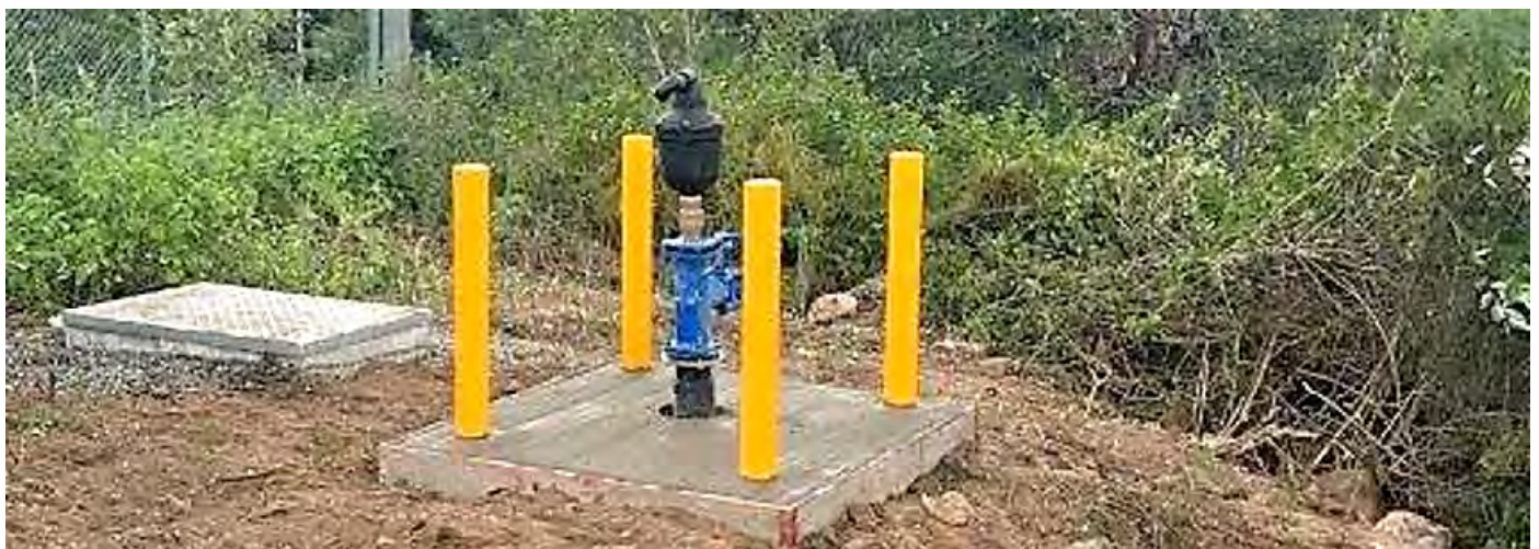
Image 2: St Lawrence Water Storage – New Air Valve installed between Plant and Supply Line
