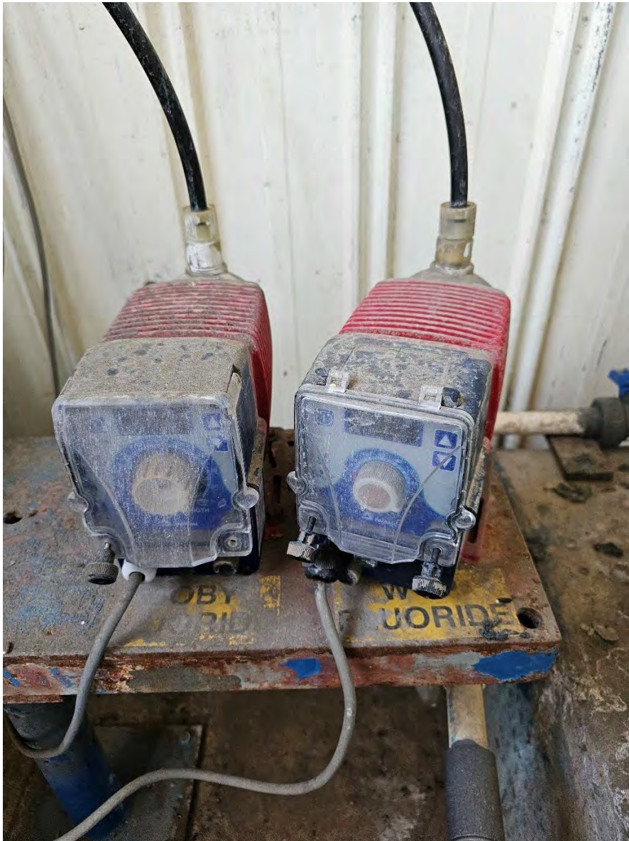
Photo 23: Moranbah WTP Fluoride Dosing Pumps – Non-Compliant with Code of Practice Item 3.2.5
