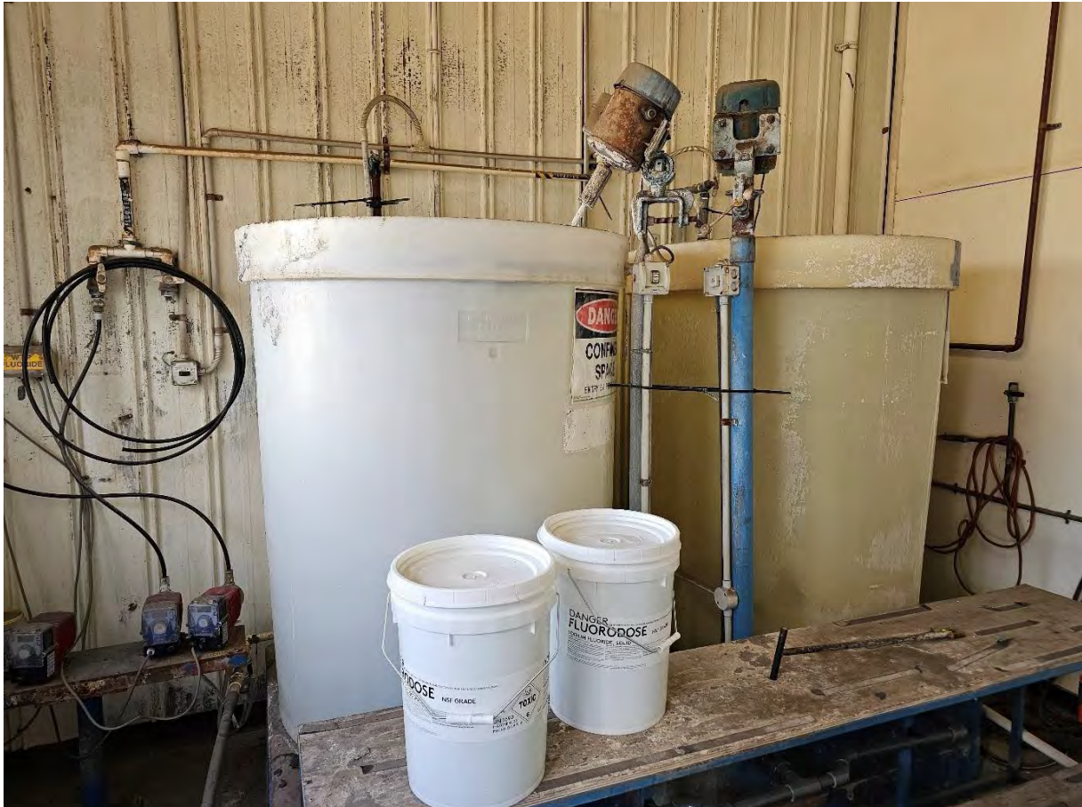
Photo 2: Moranbah WTP Fluoride Batching System
