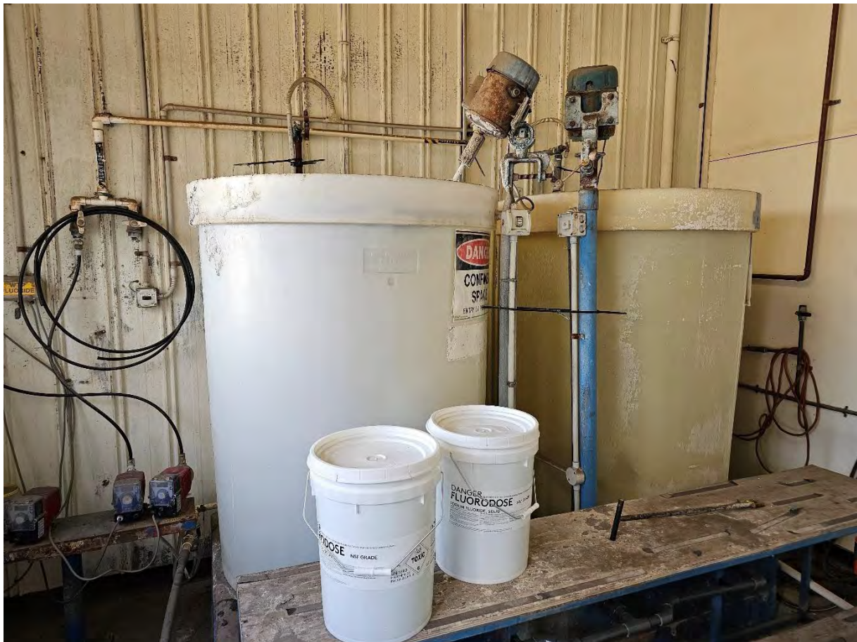
Photo 31: Moranbah WTP Dosing Pumps Hardwired – Compliant with Code of Practice Item 3.8.3
