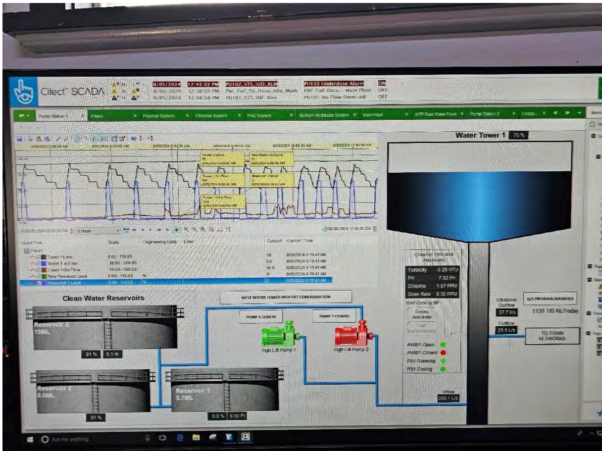
Photo 6: Moranbah WTP – Treated Water SCADA Page
