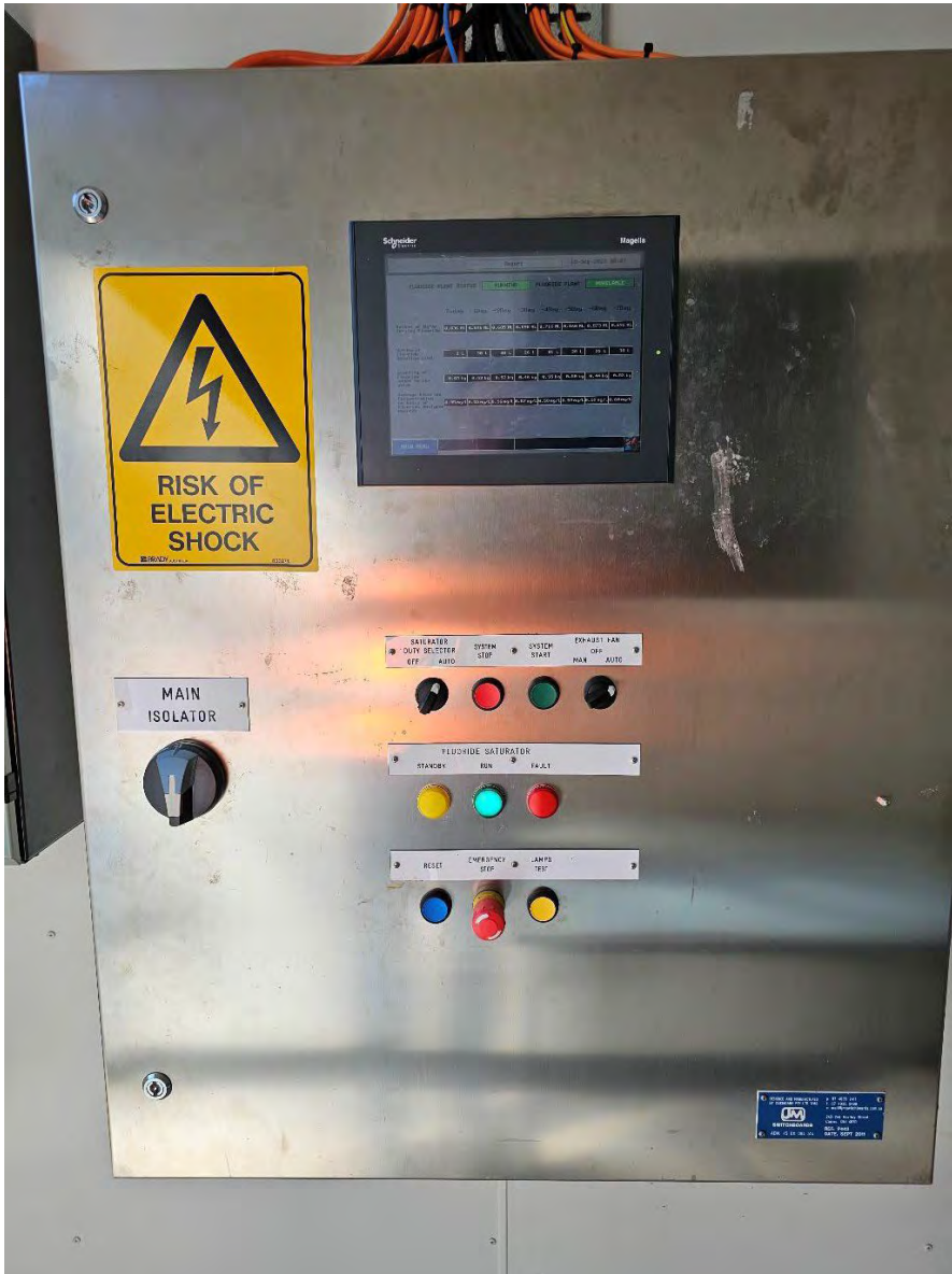
Photo 38: Tieri WTP Fluoride Switchboard Control Panel
