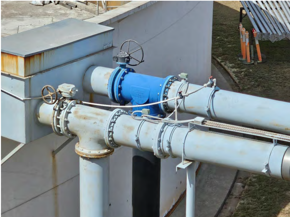
Photo 17: Filtered Water Flowmeters should be installed upstream of Fluoride Dosing Point on each pipeline (from Main Plant and Boby Plant).
