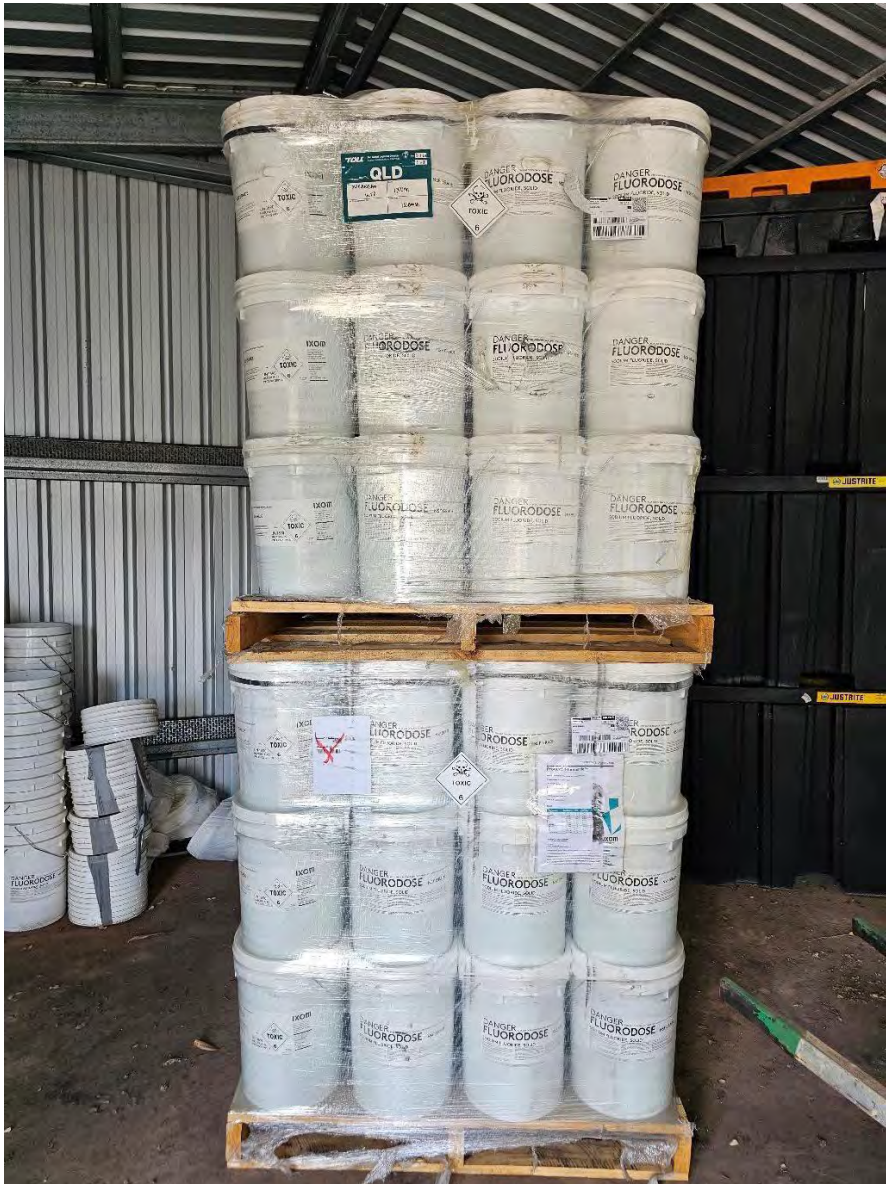
Photo 21: Moranbah WTP Fluoride Storage – Compliant with Code of Practice Item 3.2.2
