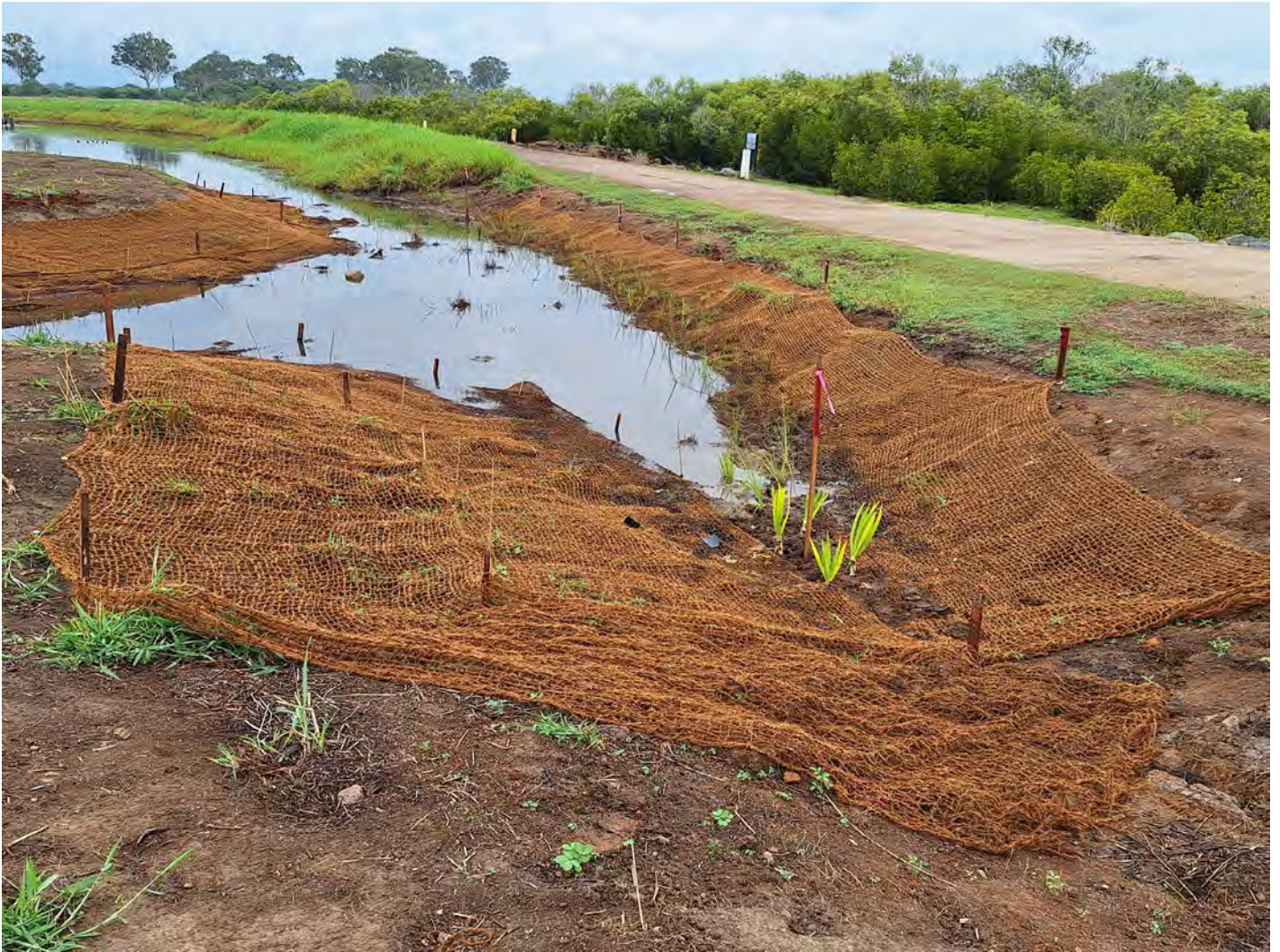
Revegetation undertaken at St. Lawrence by Koinmerburra Aboriginal Corporation after hymenachne removal
