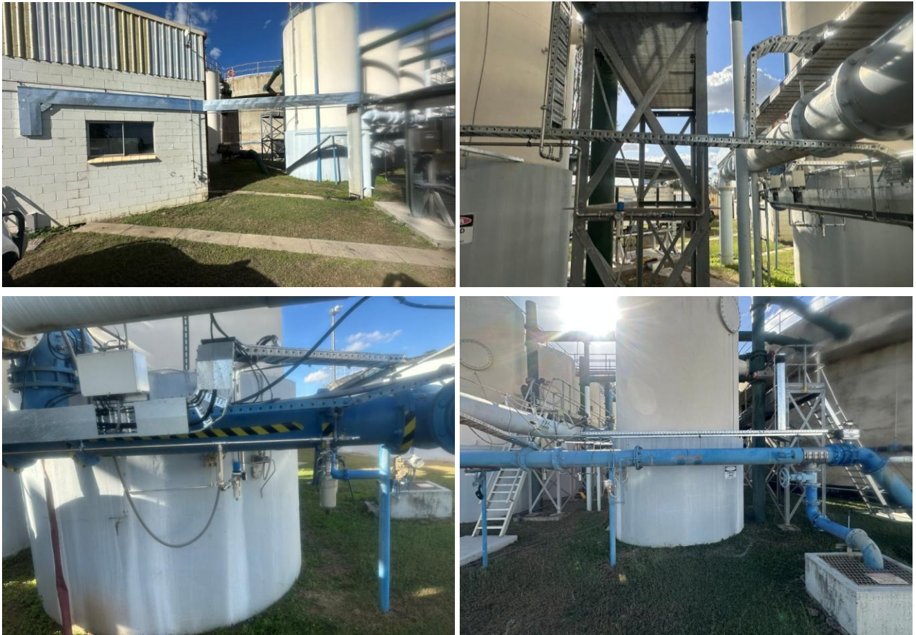
Image 4: MBH Main WTP air lines and valves to Filters 1 – 9
