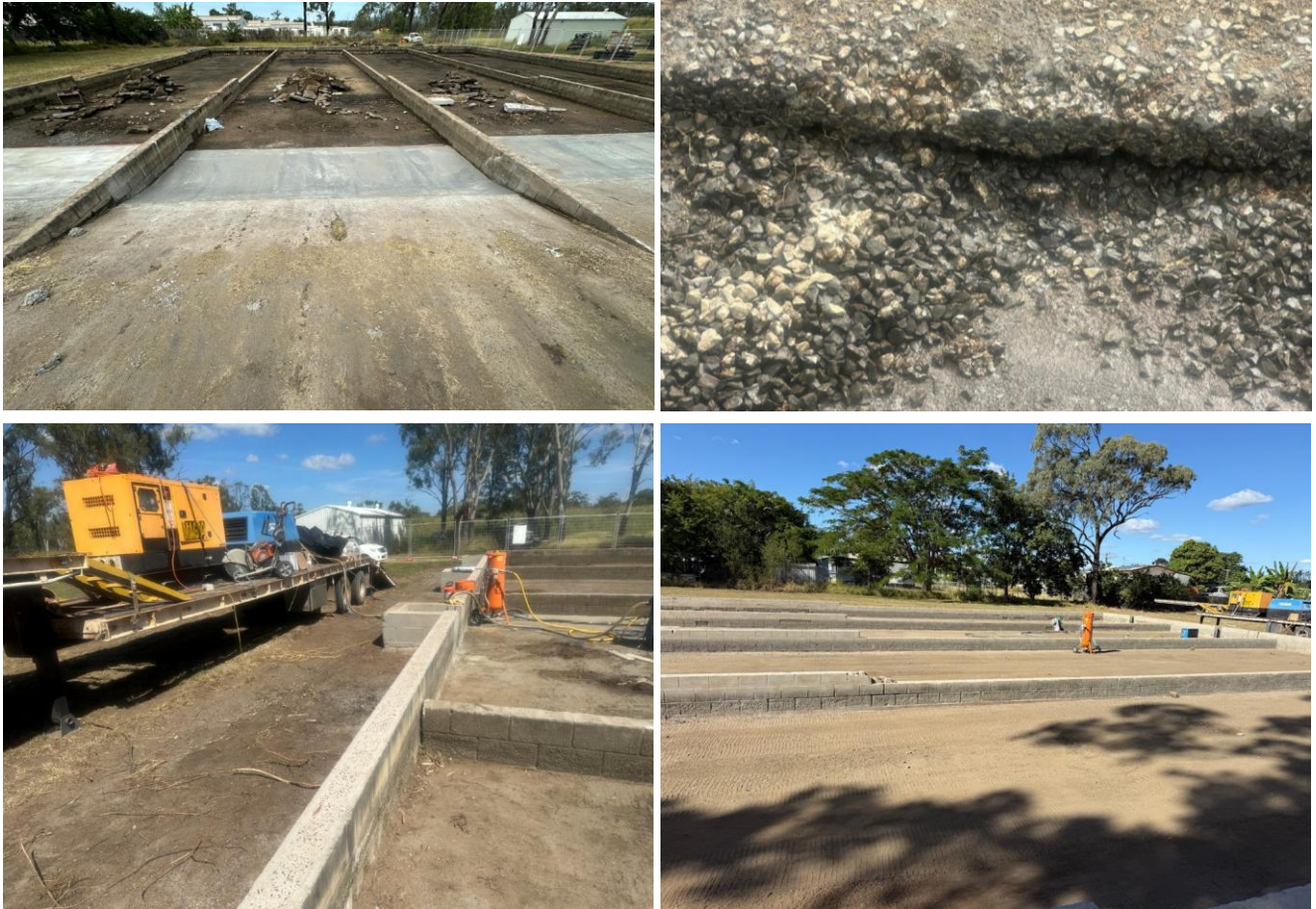
Image 5: Dysart WTP Drying Beds
