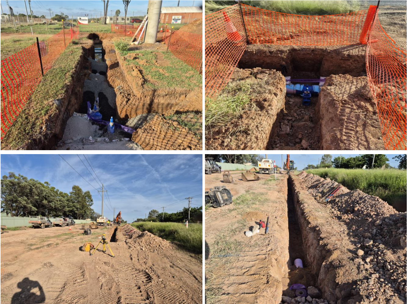
Image 1: MBH Recycled Water Network - Irrigation pipeline installation along Goonyella Road for Sarchedon Drive
