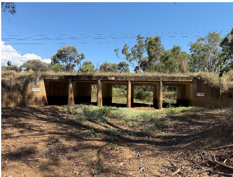
Figure 4-3 Queensland Rail 5 x 3.0 m x 3.2 m Measured Box Culverts
